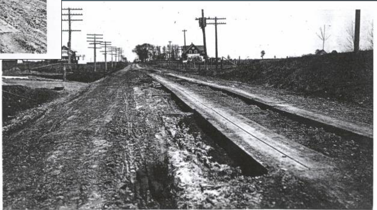
Planks covering mud holes on Grand Avenue, north of Ames, 1920. (Courtesy: Iowa State Highway Commission)
