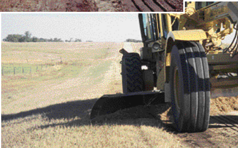
The material from the high shoulder is then pulled into the cut that has just been made. Generally, this material will have to be worked several times with the grader to break it up enough to spread evenly.
