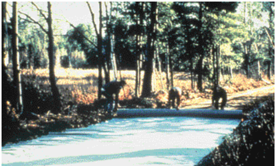
A decision was made to stabilize the above road. A road crew is shown rolling out a fabric over the existing road surface.
