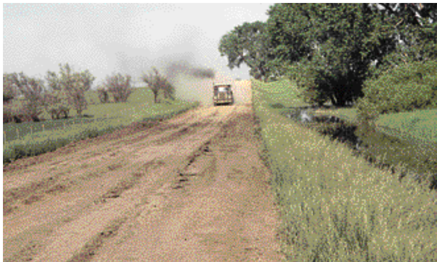
This road has been badly damaged from a heavy haul. It would be useless to begin hauling and placing fresh gravel until the entire roadway has been reshaped.
